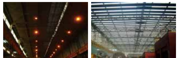
Increase of interior illumination to 500Lx from existing 80Lx by installing natural lighting windows (daytime)
