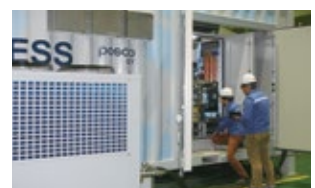
↑ POSCO ICT's Pohang ESS Test Center (144MW)
