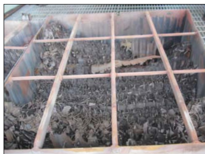
Severe corrosion of the heating elements (ordinary commercial sulfuric acid corrosion resistant steel)
